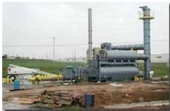
Small plant for waste-water recycling
